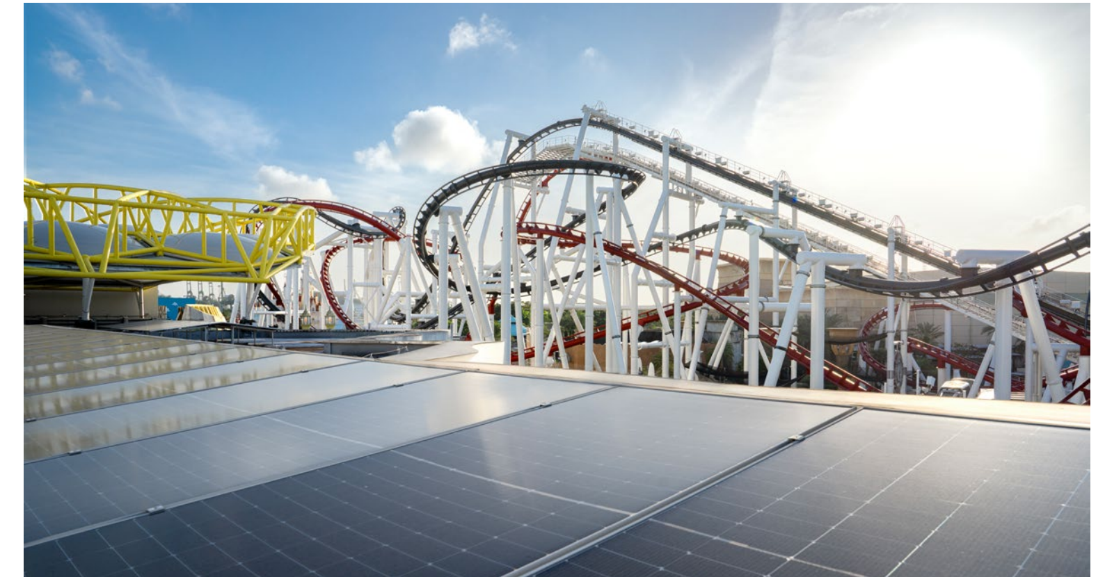
Universal Studios Singapore rooftop solar panels
