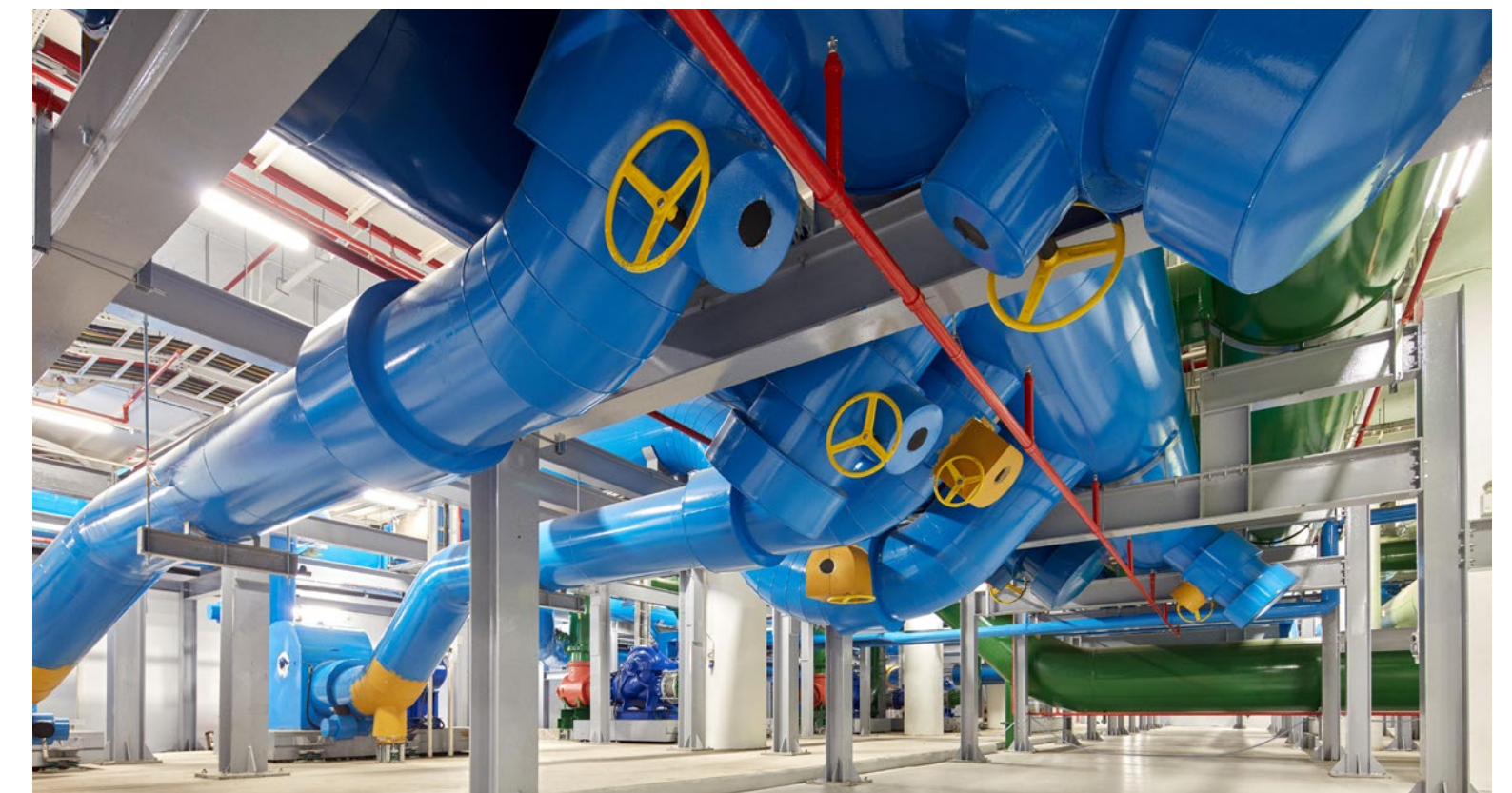
High-efficiency District Cooling Plant (DCP)
