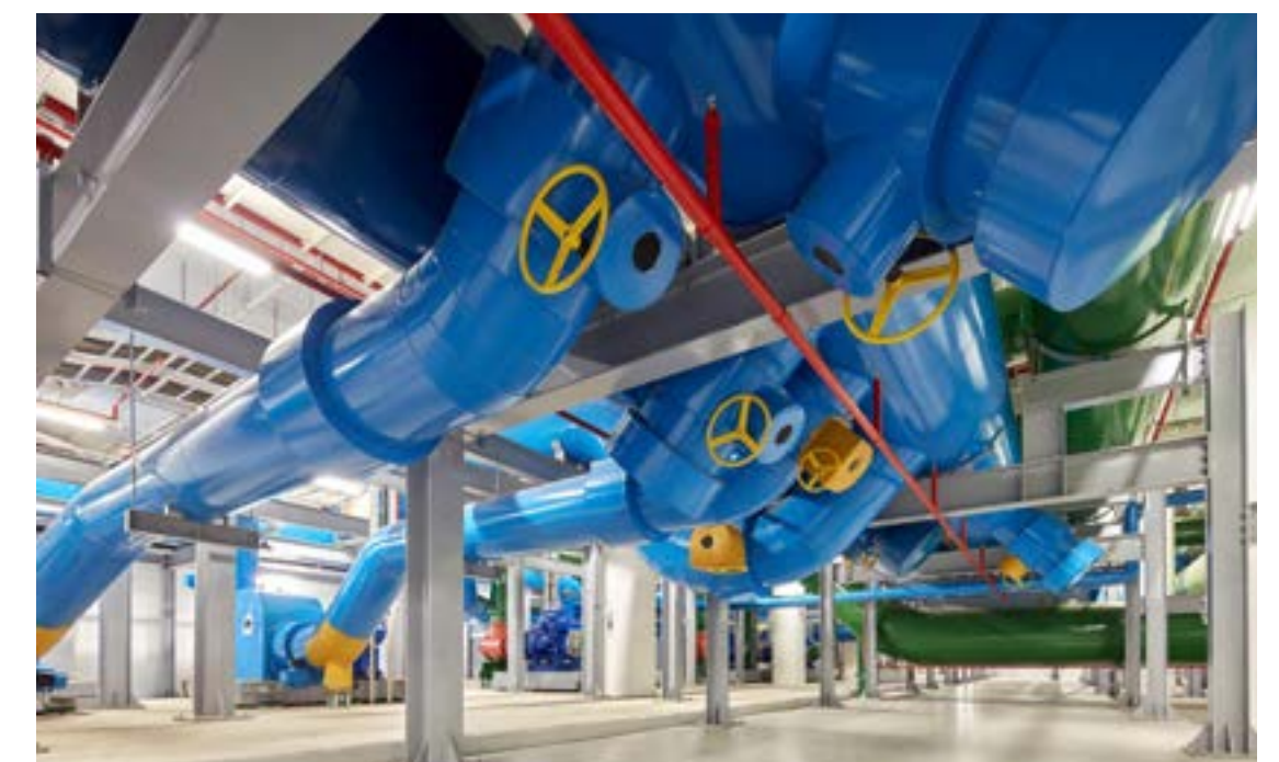
DCP 2.0 situated in RWS
